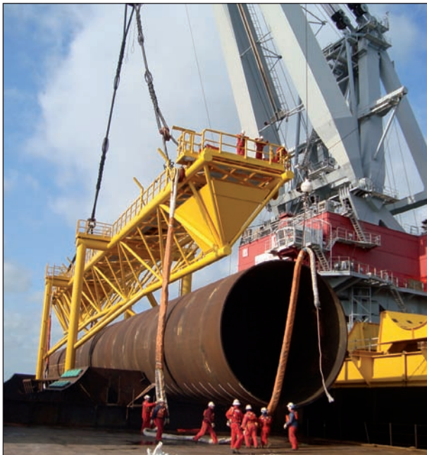
Seaway Heavy Lifting's Stanislav Yudin employed heavy lift slings made of Samson's 144mm diameter AmSteel-Blue to install 140 monopiles for the Greater Gabbard wind farm development in the North Sea.
